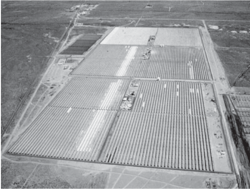
Figure 13.13 Large array of parabolic troughs for electric power generation.
