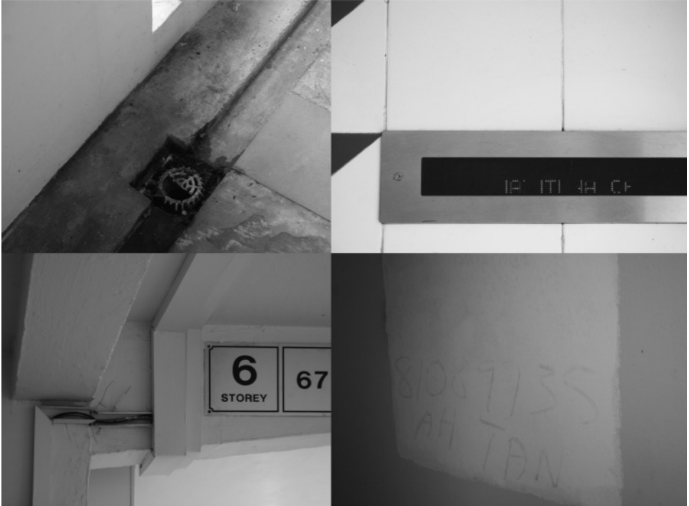
Figure 8.3 Defects at Block 22, Bukit Ho Swee. Authors' photo.
