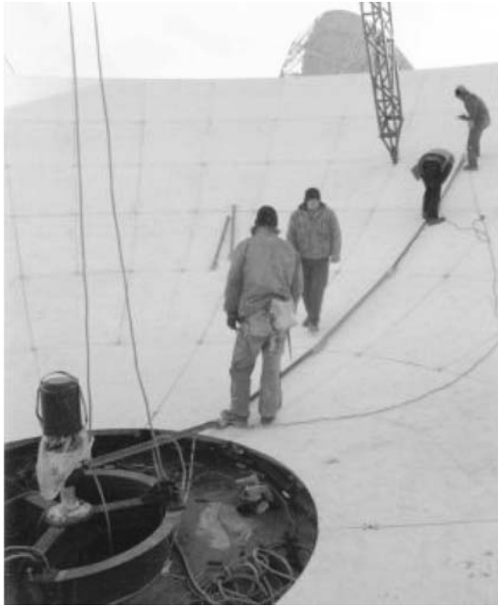
Figure 9. Linkage sets alignment hole drilling for targets from theodolite at dish center.
