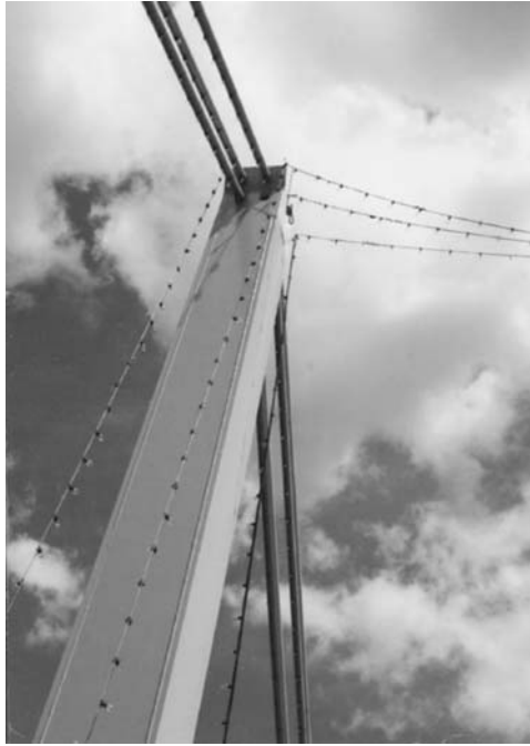
Figure 7.20 Close-up view of the upright column with a missing tie rod 1
