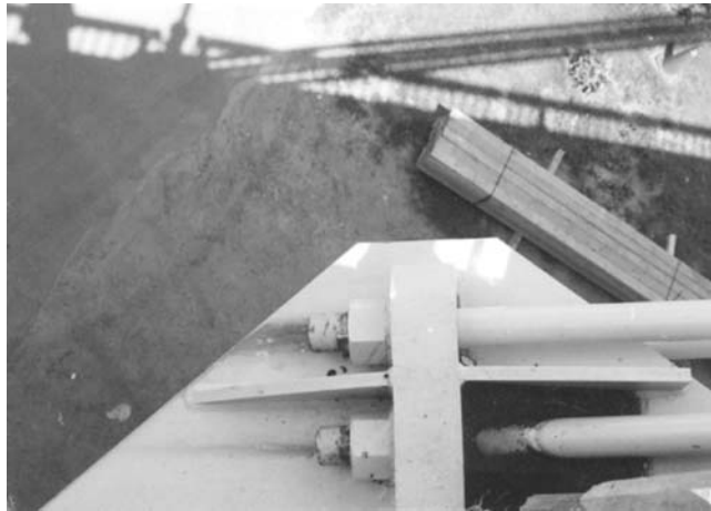
Figure 7.19 Close-up view of the exposed tie rods; corrosion of the unpainted exposed areas may be noted 1
