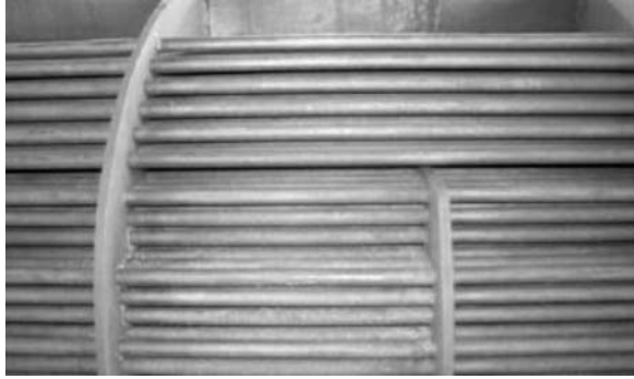
Figure 7.31 GE3B tube outside surface shows no corrosion or pitting 1
