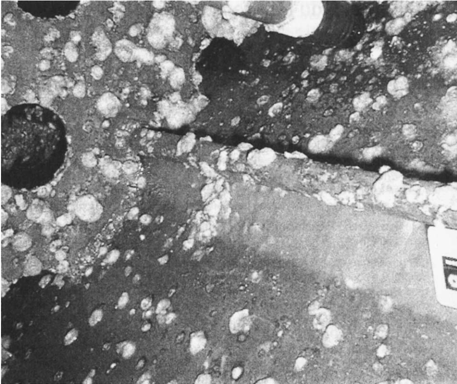
Figure D.1.15. Aspect of pitting in a tank with stagnant water.
