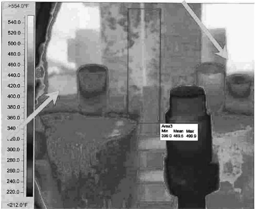
Figure 17-19. A thermal image of the casing while the unit was running. The arrows point at the area of bolt replacement.
