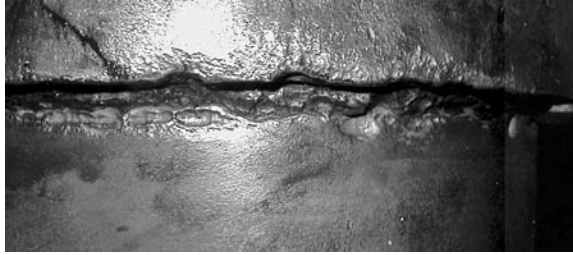
PHOTO 7.15 Pitting corrosion adjacent to the weld on a steel elevator cylinder — caused by the residual stress.
