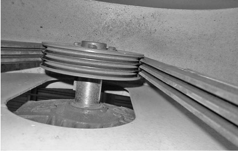
PHOTO 9.3 The cover separation on the right side of the sheave is obvious. This is the result of improper installation procedures.
