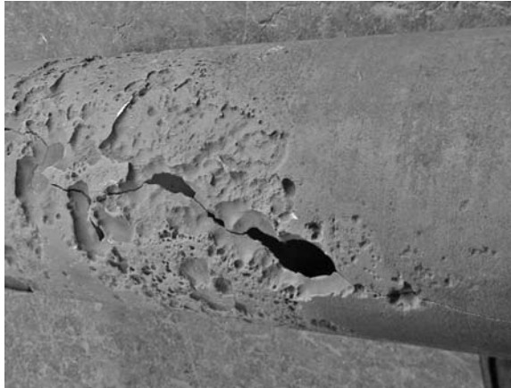
PHOTO 7.8 Selective leaching of a buried pipe.
