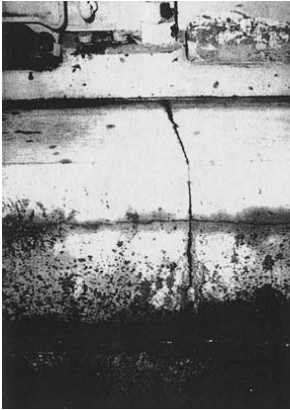
Figure 3-4. A photograph showing foundation cracks at an anchor bolt. This crack is in a plane perpendicular to the crankshaft.
