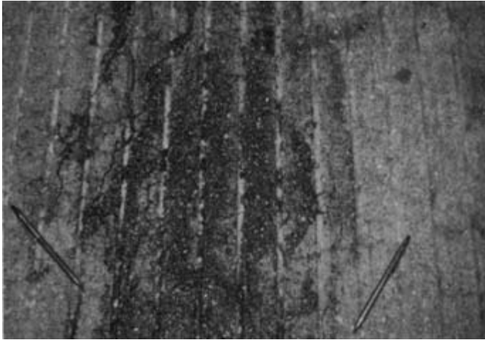
Figure 3-2. Hairline curing cracks become visible as the solvent in Figure 3-1 evaporates from the surface (courtesy of Adhesive Services Company).
