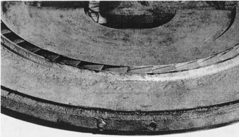
Figure 8-28. Turbine diaphragm for the casing shown in Figure 8-27. Steam erosion, which is very evident on the outer diameter, is repaired by welding. Nozzles can also be repaired, although these are in good condition.
