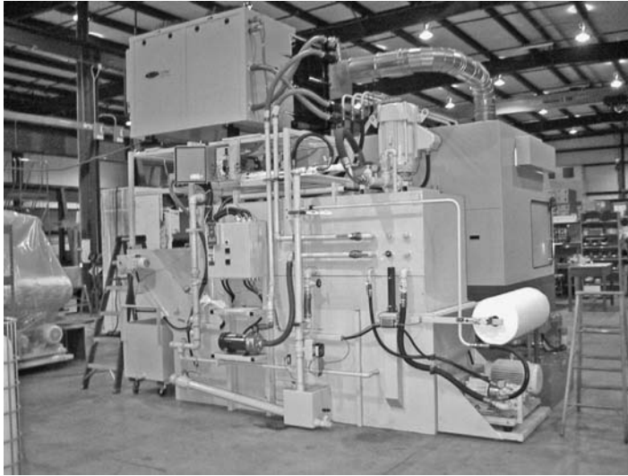
FIGURE 16.16 Oil coolant system for use with a 40-Hp grinder operating with plated CBN wheels (pumps, chiller, filter, settling tank, and mist collection). (Courtesy of Campbell Grinders, Spring Lake, MI. With permission.)
