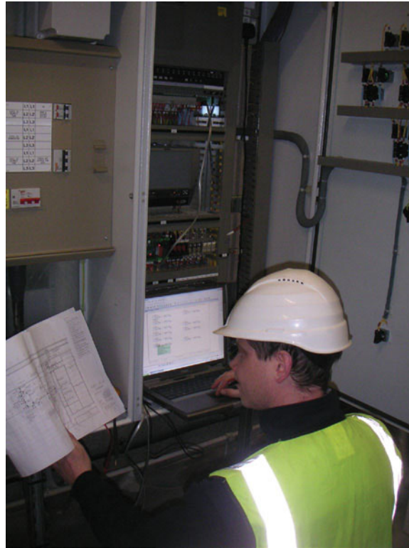
Figure 10.6 Specialist BEMS contractor
