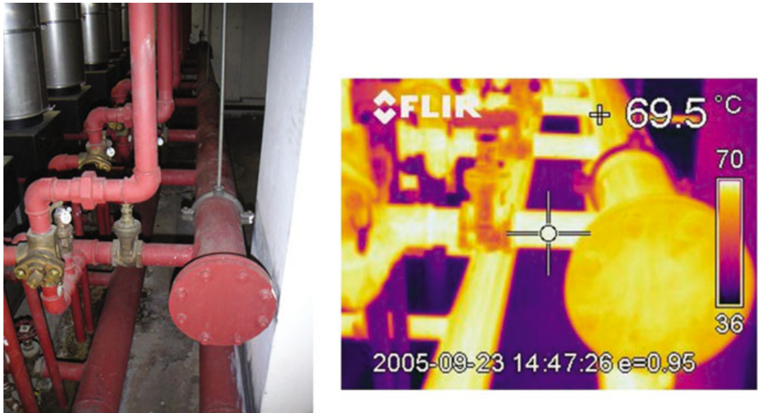
Figure T12.13 Back of boiler pipework – insulation needed!
