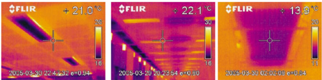
Panels in centre of picture are not functioning
