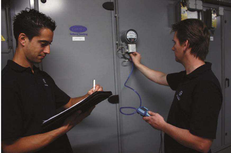
Figure 11.7 Commissioning inspection and validation – check of pressure gauge and airflow
