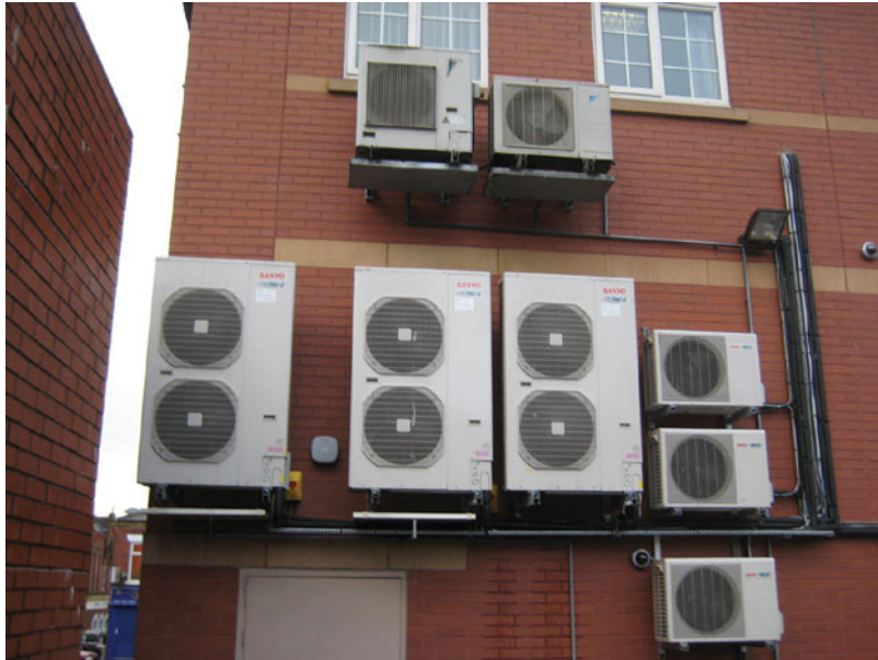
Figure 9.12 A wall of split condenser units
