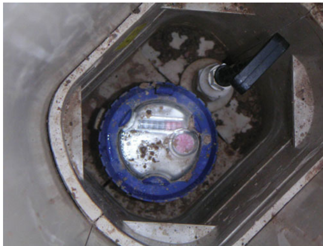
Figure 7.1 A water meter; often out of sight, out of mind
