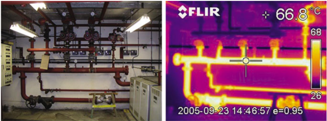
Figure T12.15 Pipework checking – insulation needed!
