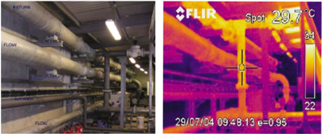
Figure T12.8 Measuring flow and return temperatures for maintenance and commissioning
