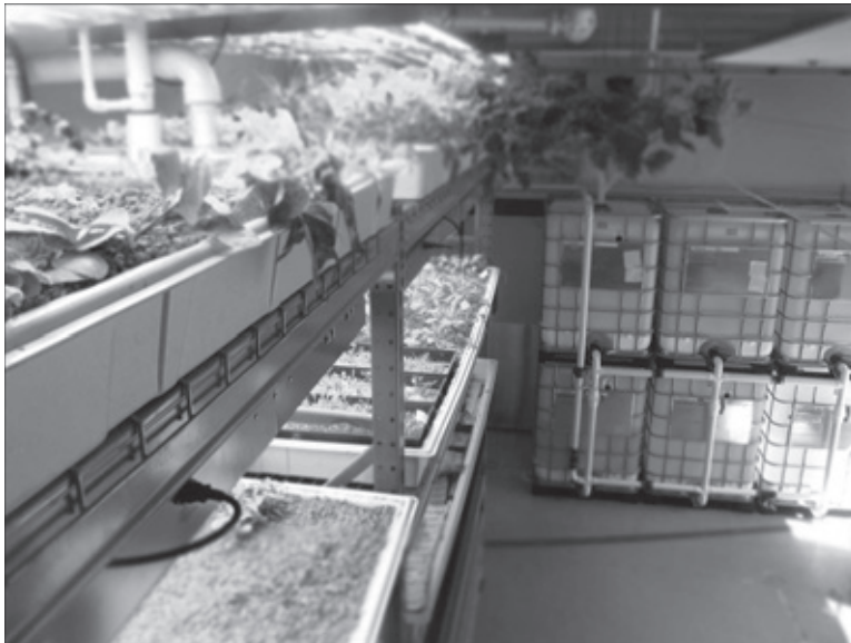
Aquaponics and rain catchment system between the kitchens at Main Event Caterers near Washington, D.C.
