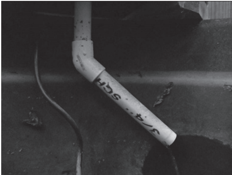
A Coanda drain beneath a grow bed. The 45-degree angle aids in forming a hydrodynamic plug to start the siphoning action for a bell siphon or internal loop siphon. The dust is an indication of how long it's worked without needing adjustment.
