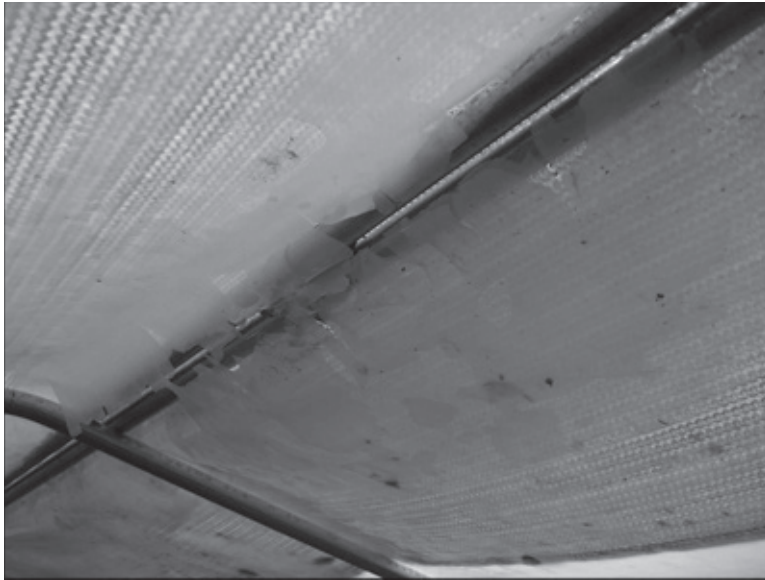
Check your system periodically so you know what you'll need to replace, like this shredded plastic roofing.
