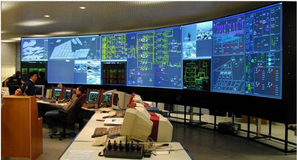
Fig. 4. Large display walls make it possible to present a plant overview for the operators.
