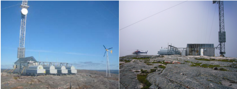
Figure 19. Telecom station of Bell-Canada at Kuujuarapik [37]
