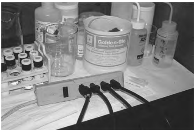
FIGURE 5.3.5.2 Outlet in Chemical Hood. A strip outlet in a chemical hood represents a fire hazard since the outlets and switch are not spark-proof and flammable chemicals are often used in hoods. The dangling cords might also present a trip hazard. A liquid spill could also present a shock hazard. (From Journal of Chemical Health and Safety 7(5): 6 (2000). Used with permission. Copyright © 2000 Division of Chemical Safety and Health of the American Chemical Society.)
