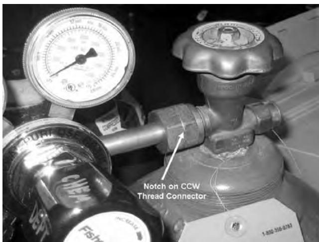
FIGURE 5.3.1.3 Notch in Connecting Nut Indicating CCW Thread. For most normal gases the CGA connector attaches clockwise (CW), but for flammable gases the CGA connector attaches counterclockwise (CCW).
