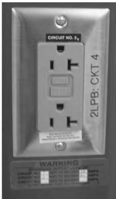
FIGURE 5.3.5.1 Ground Fault Circuit Interrupter (GFCI). These outlets are required at any location near water sources or sinks, although older laboratories may not have these if they have not been upgraded to meet current electrical codes.
